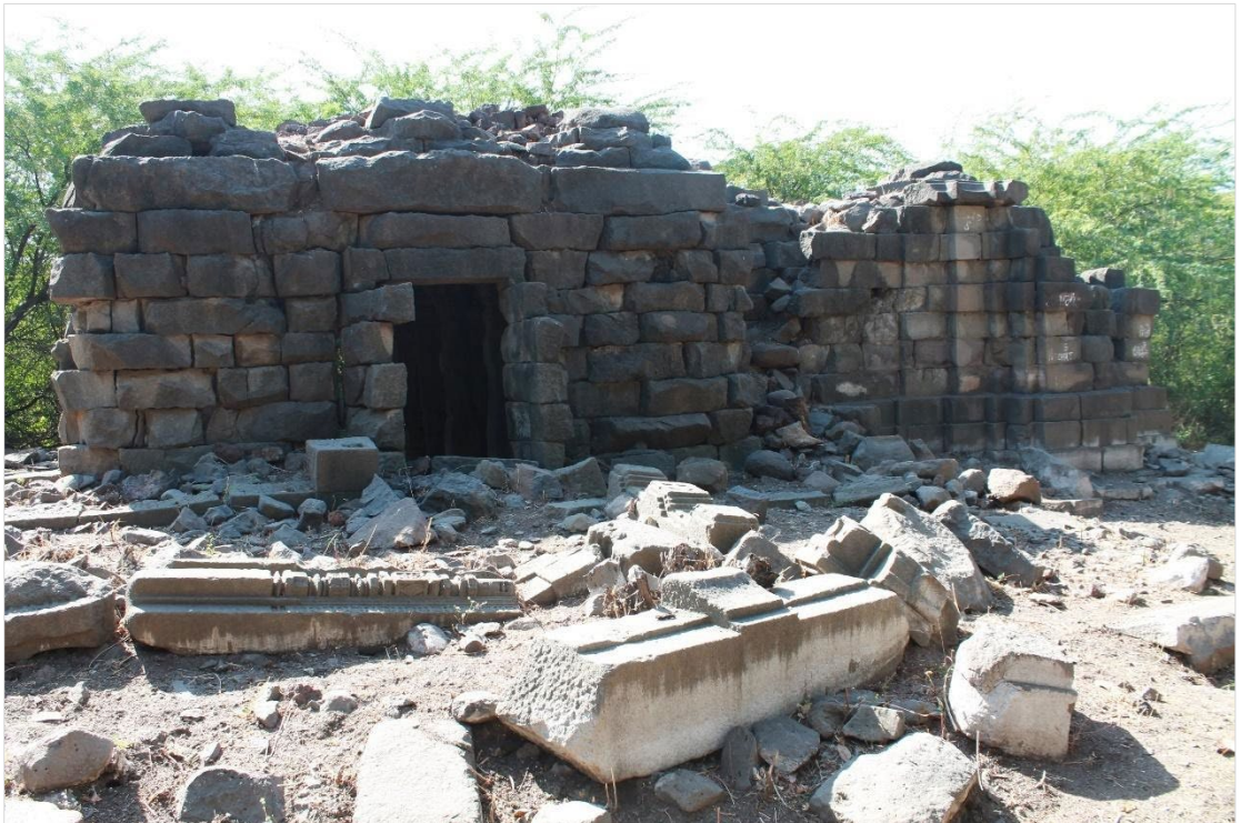
Fig. 3.77: South-elevation of Copadā temple – Maṇḍapa and extended plinth are in dilapidated state
